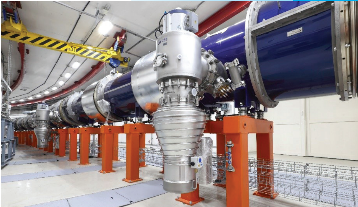
Tunnel of the NICA collider
